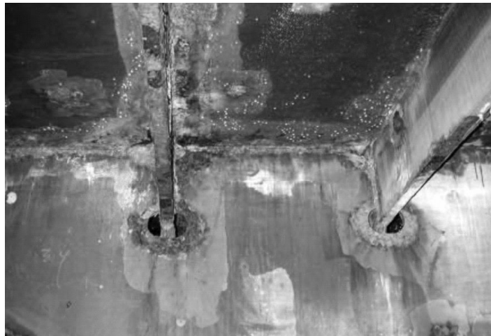
Fig. 1 Heavily corroded under-deck of 20 years old oil tanker
